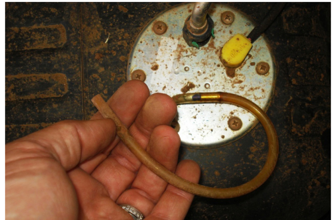
Figure 11. Vent from the top of the tank through a short opaque tube.
